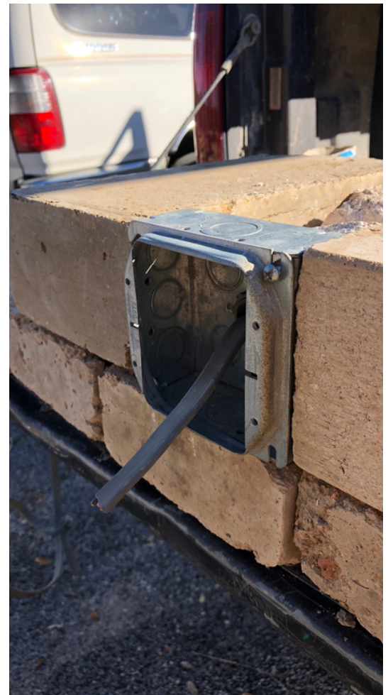
Electrical box placed in the wall during construction with conduit placed between the two wythes of blocks.
