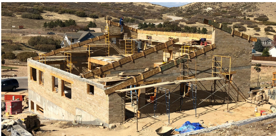
Exterior walls under construction with formwork for poured, reinforced concrete bond beam at the top of the wall and between floor levels.
